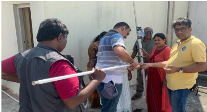
VU3CJM, VU3FTW, VU3UBN, VU3FCE, VU3LXI and VU2FI assembling the X50 VHF/UHF antenna for the installation.
