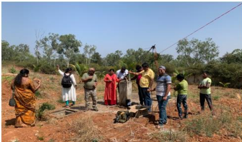
VU3LXI, VU3DUG, VU2FI, VU3FCE, VU3CJM, VU3UBN and VU3FTW along with school students and teacher doing the installation of Inverted-V HF antenna using the indigenously assembled INSTAMAST.
